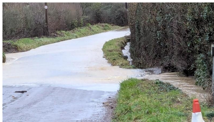
Immediate Area Flooding Jarmany Hill, looking east towards the site, 27 Jan 2026
